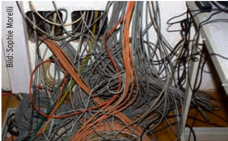
Image from the self-maintained datacenter at servus.at
